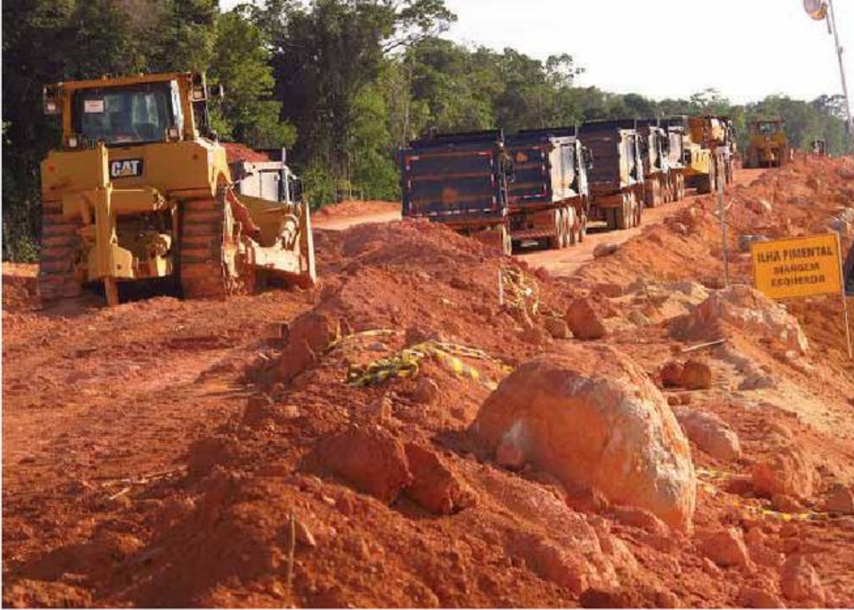
Left: Construction has begun with the opening of new roads through the virgin forests.
