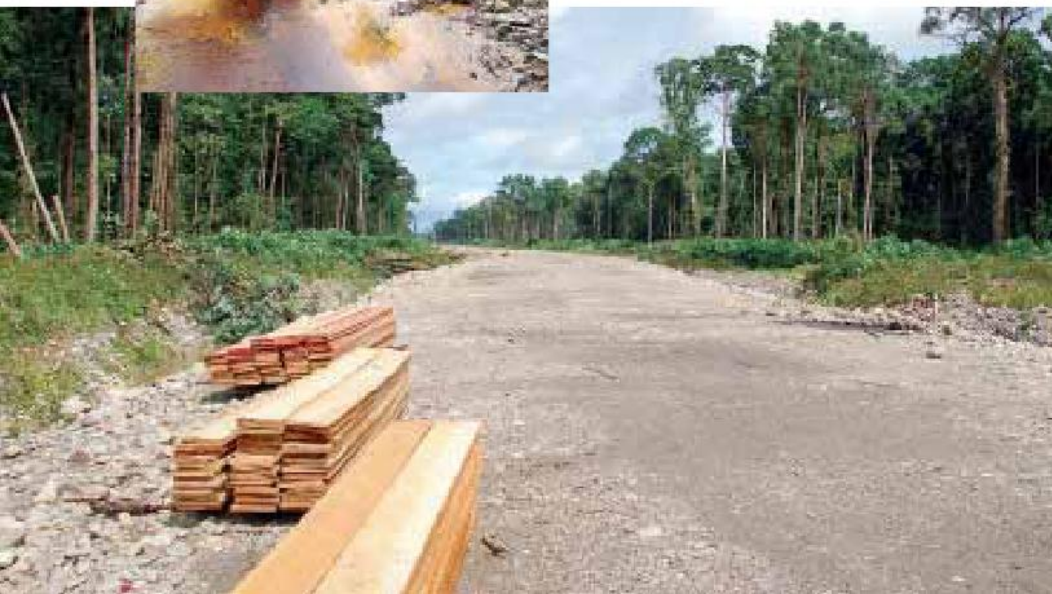
Opposite page: The broad Wataikwa River can be reached via the new road. In a few years there will be a bridge over the river here—and a route to the mountains of the Great Dividing Range, visible on the horizon.
